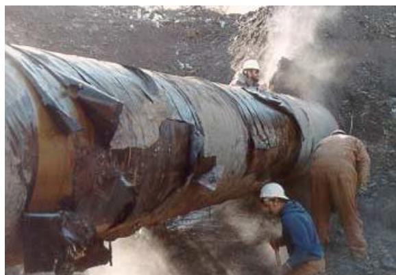
Fig. 2 Gas and Liquid Transmission Pipeline Corrosion under Insulation [19].
